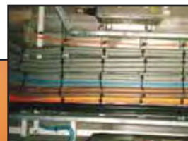
Marine Cable Bundling
